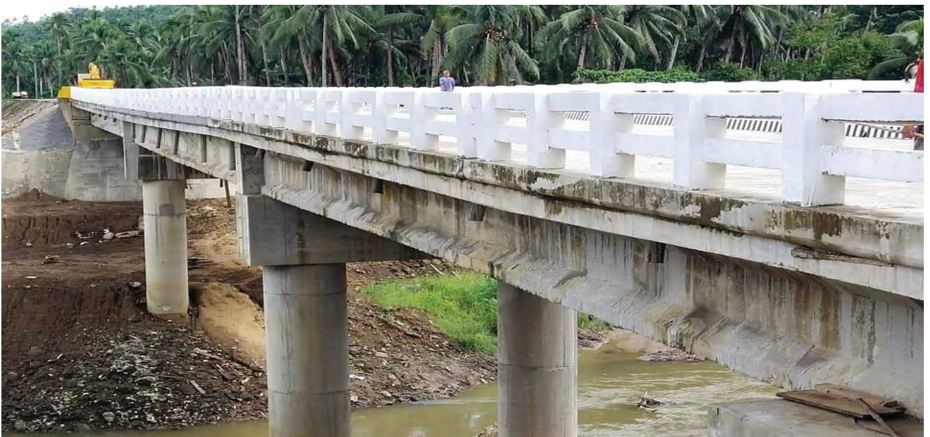
The Php 98.5M 12km Lope de Vega – Silvino Lobos Road (Lope de Vega Section) in Northern Samar Province at 100% completion. This road connects the Municipalities of Silvino Lobos and Lope de Vega in the Eastern Visayas Region.
